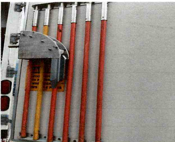
Figura NO.15 pole assy , tool instaladas
